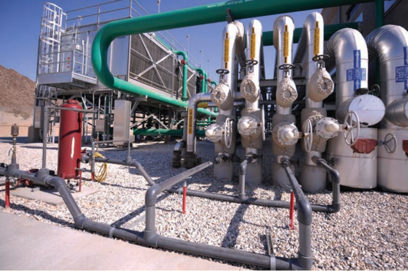
At 9.2 megawatts (MW), the new CHP system at the Marine Corps Air Ground Combat Center in Twentynine Palms, California, is the largest of its kind in the Marine Corps.
