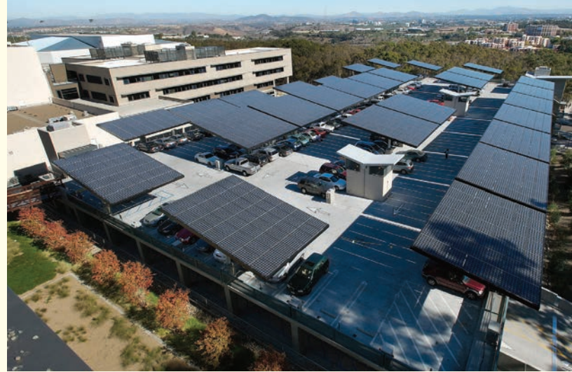
Solar canopies atop University of California, San Diego's Hopkins Garage includes 1.2MW of solar photovoltaics.
